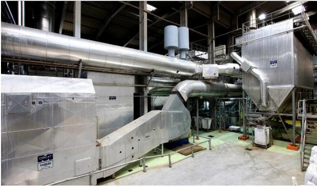
▲ Cooperl – digestate valorisation facilities
